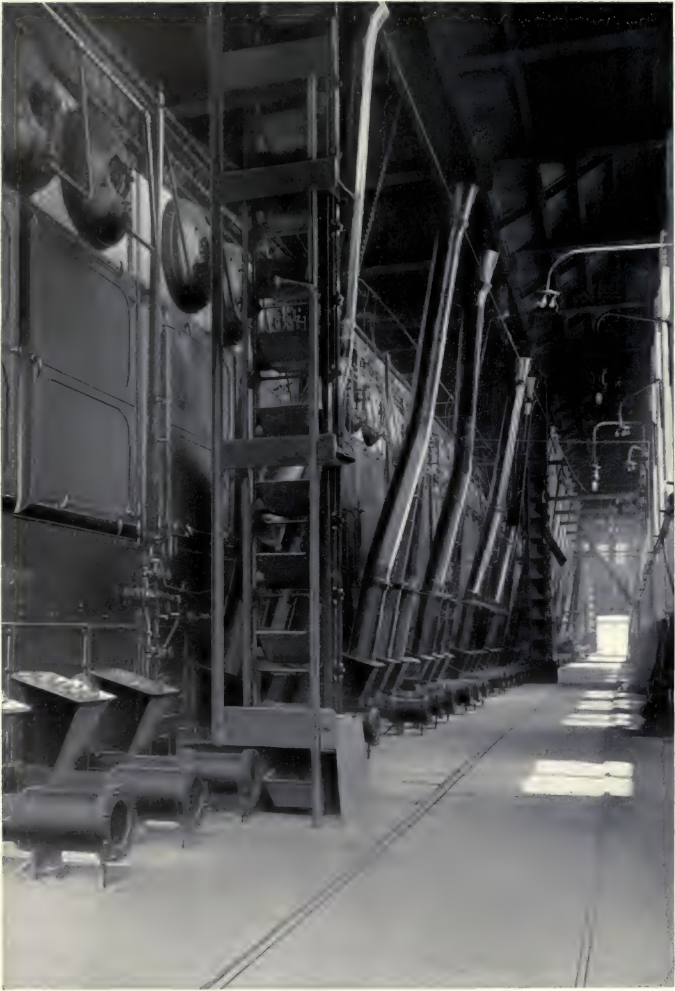
GEORGIA RAILWAY & POWER CO., ATLANTA, GA. BUTLER STREET STATION BABCOCK & WILCOX SUPERHEATERS INSTALLED IN 8400 HORSE POWER OF BABCOCK & WILCOX BOILERS
